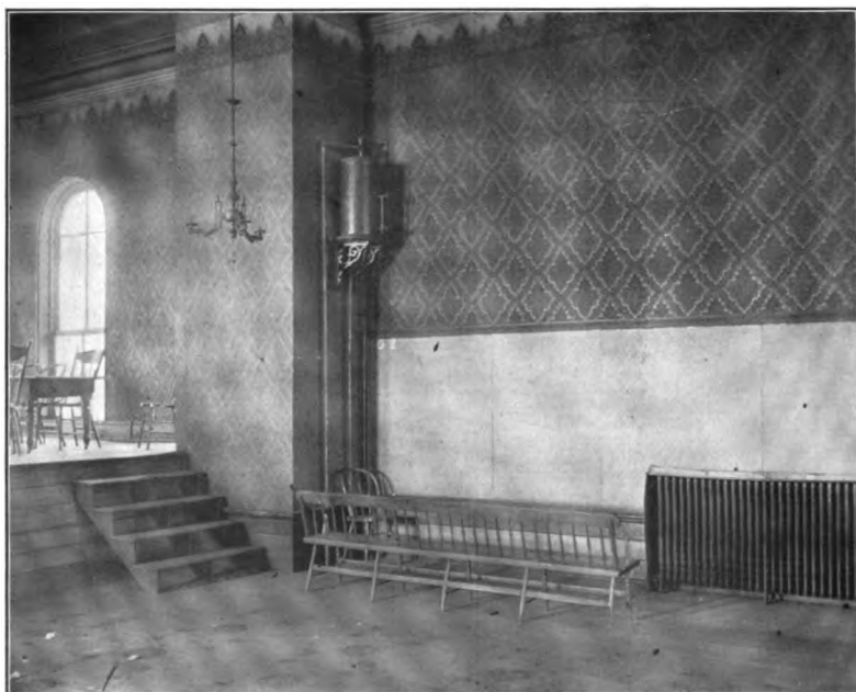
Detail of Assembly Room. This assembly room was a veritable death trap, just over the boiler room. It was given up following the Cleveland fire.
