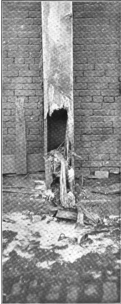
WOODEN CHUTE FROM A SECOND-STORY GALLERY Dumping its filth at the curb on Carson Street
